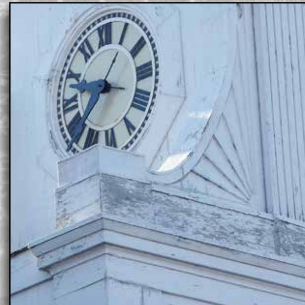
ORIGINAL PARTS IN NEED OF RESTORATION
